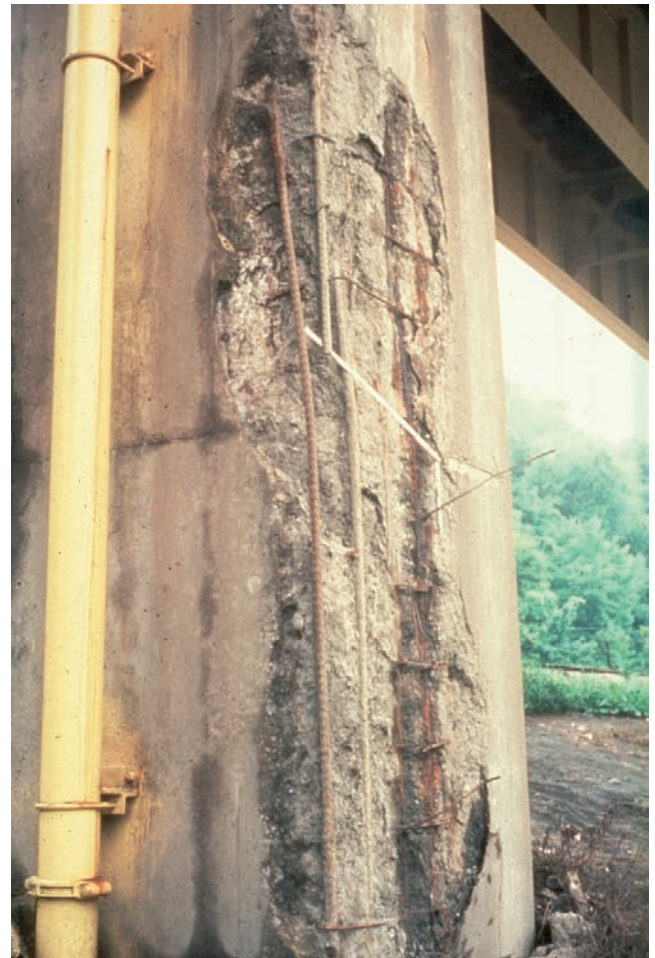
Figure 10.2.36 Concrete Deterioration due to Contaminated Drainage
