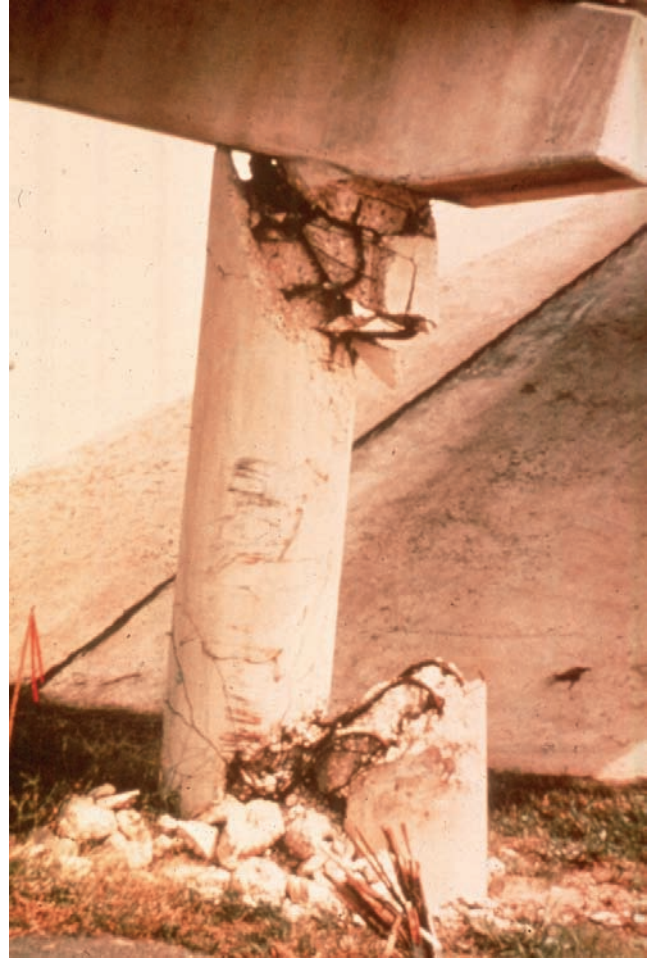
Figure 10.2.39 Collision Damage to Pier Column
