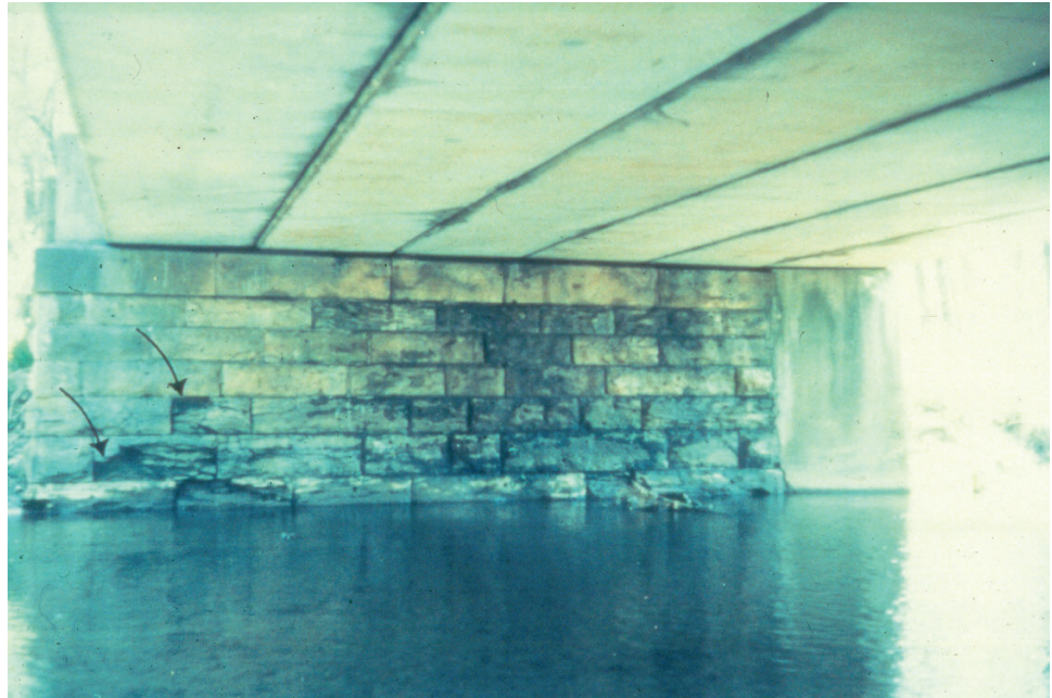
Figure 10.2.51 Deteriorated and Missing Stone at Masonry Pier
