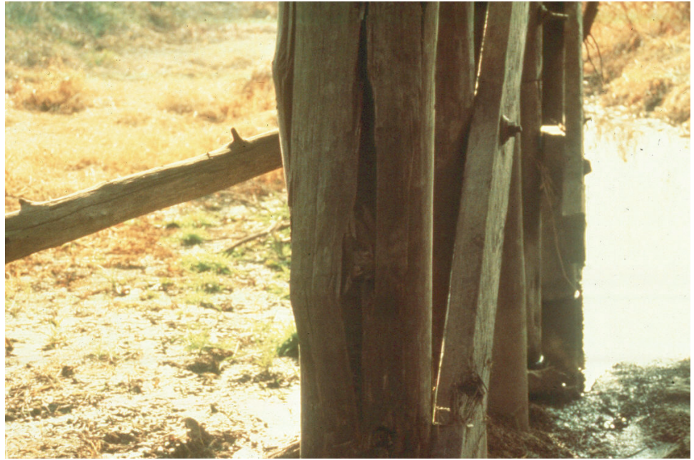
Figure 10.2.48 Timber Pile Bent with Partial “Brooming” Failure at First Pile
