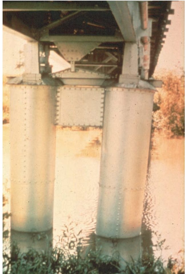
Figure 10.2.35 Tipping of Bent due to Scour/Undermining
