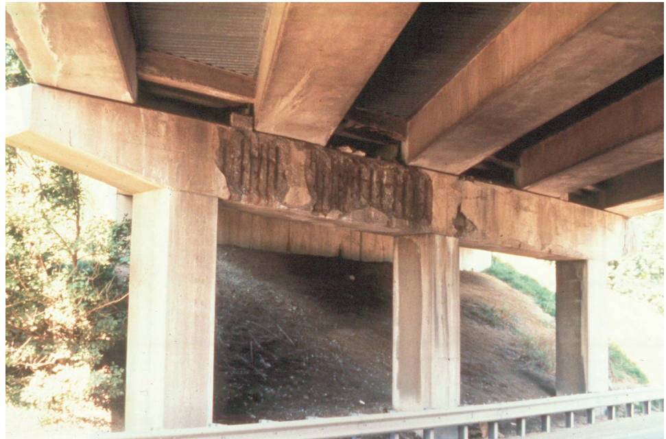
Figure 10.2.38 Severe Concrete Spalling on Bent Cap
