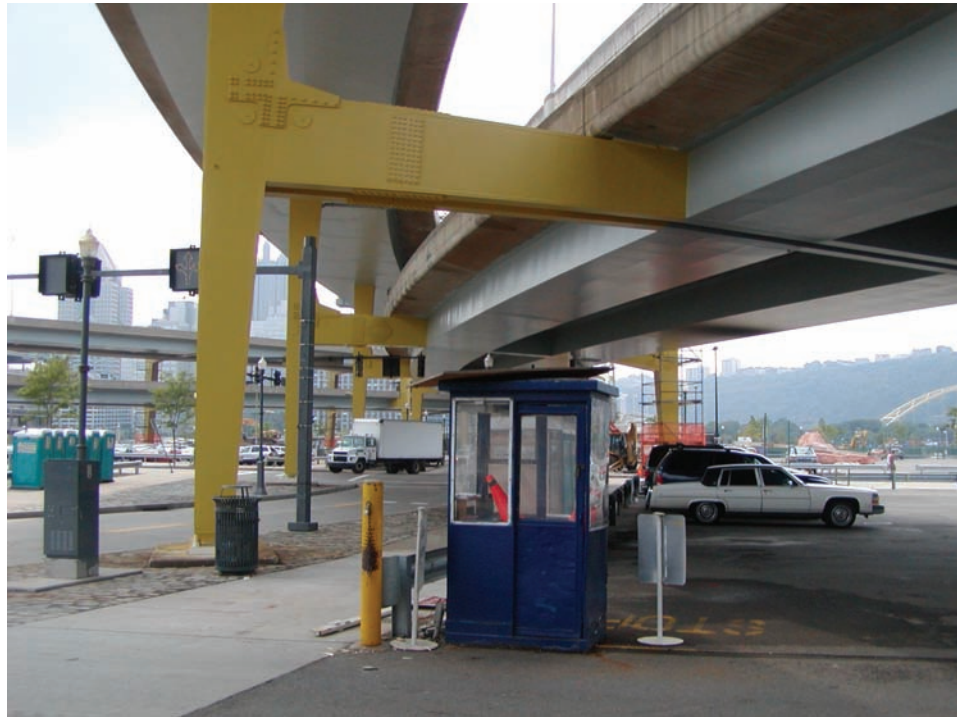
Figure 10.2.52 Fracture Critical Steel Bent
