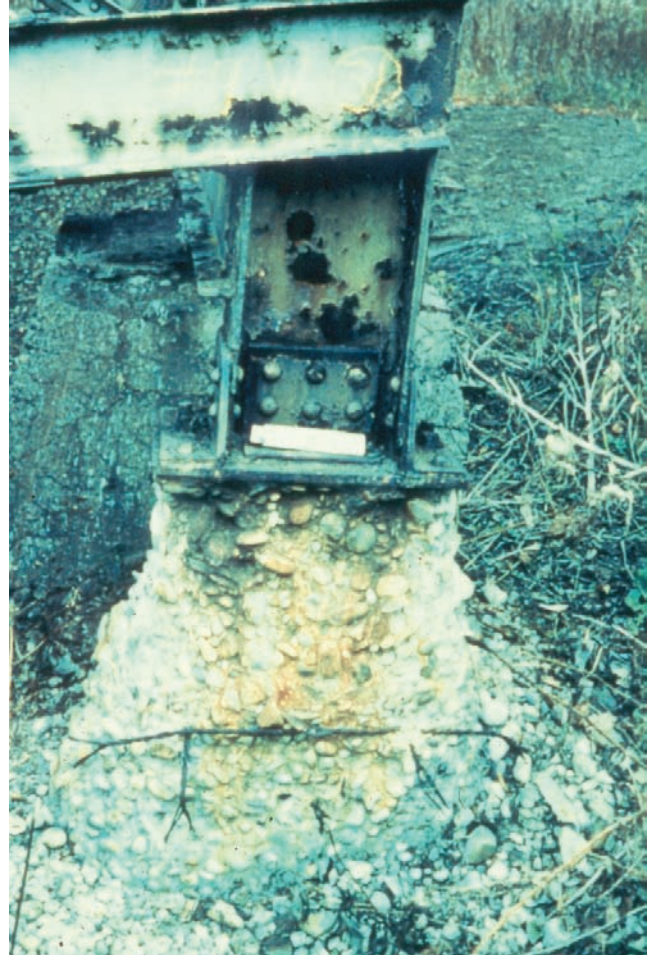
Figure 10.2.40 Deterioration of Concrete Pedestal Supporting Steel Column
