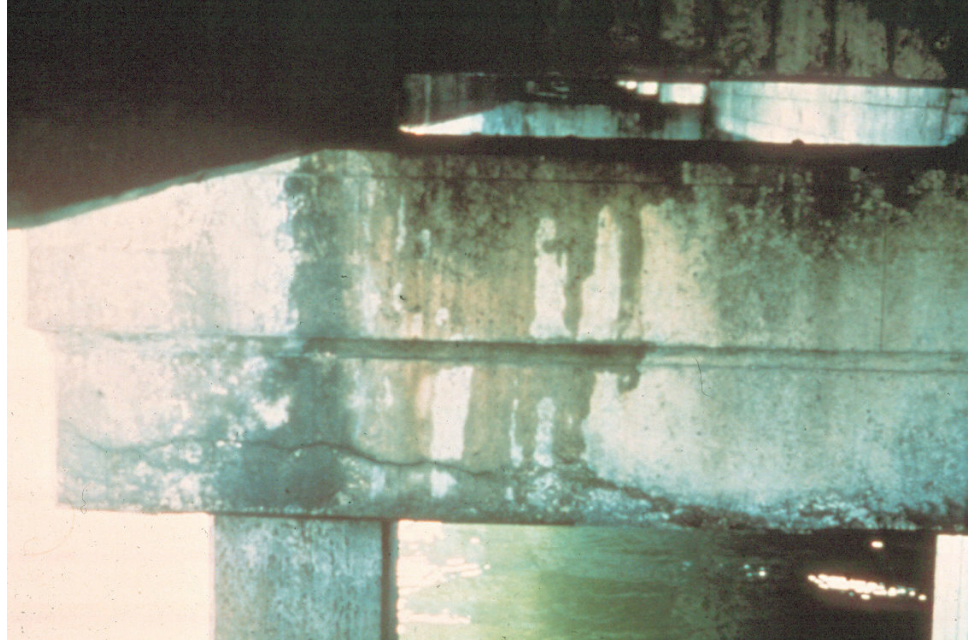
Figure 10.2.37 Crack in Concrete Bent Cap
